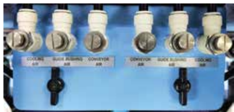
Centralized compress air controls
